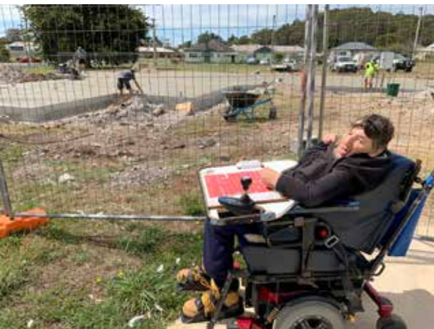
Ken visiting the site of his future home on the day they poured the slab
